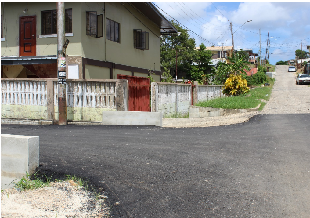
Above: Minister Hosein and officials of the RDC observe road rehabilitation works on Clark Street. Left: The construction at Clark Street St. Madeleine also included a culvert crossing.
